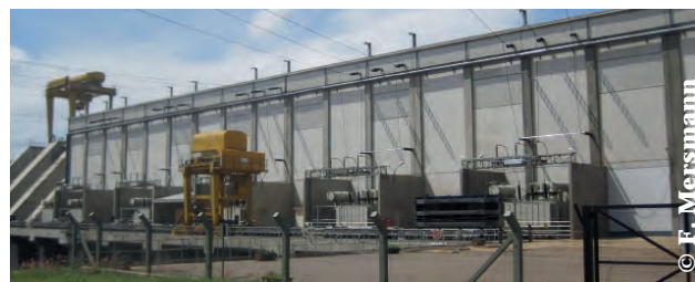
The Bujagali dam supplies about half of Uganda's electricity.
